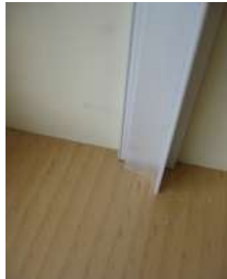
bottom of side tracks - note translucent "Z" flexible plastic weatherstrip that bears on edge of shade. Edge of shade slotted to accept "leg" of the plastic "T"
